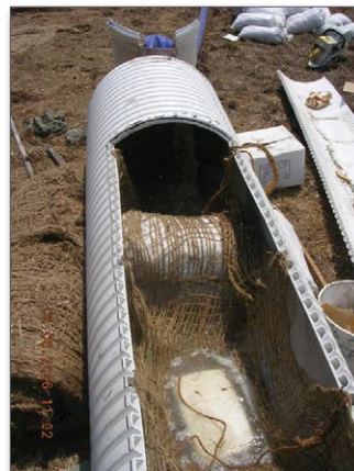
Figure 20. Split pipe with polymer blocks
