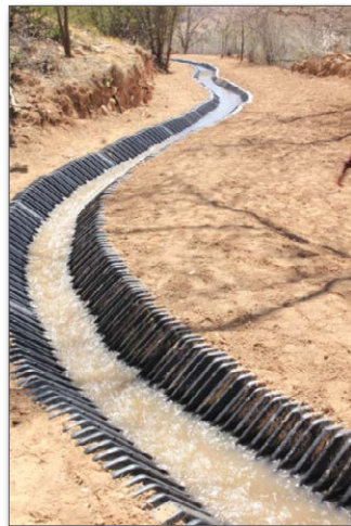
Figure 18. In-ground treatment ditch
