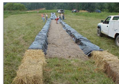
Figure 15. Lower portion of the treatment ditch
