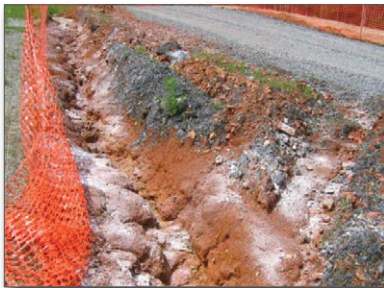
Figure 38. Eroding gully on a construction site
