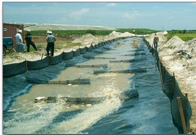
Figure 16. Flocculation ditch with checks to increase the polymer mixing
