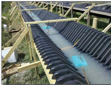
Figure 17. HDPE treatment ditch liner
